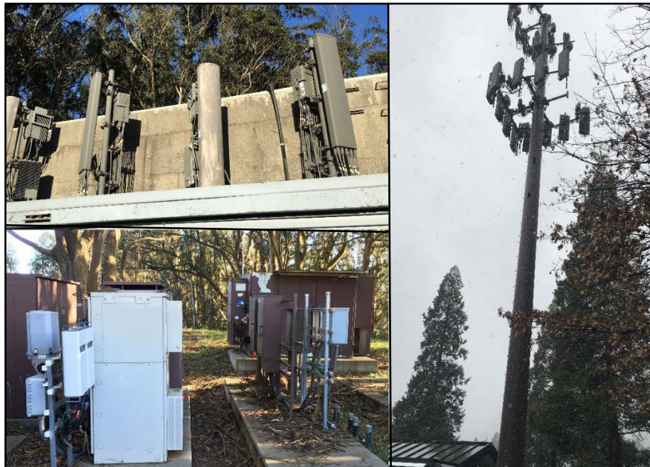
Figure 1. Examples of commercial cellular facilities on NPS land. Source: OIG.
