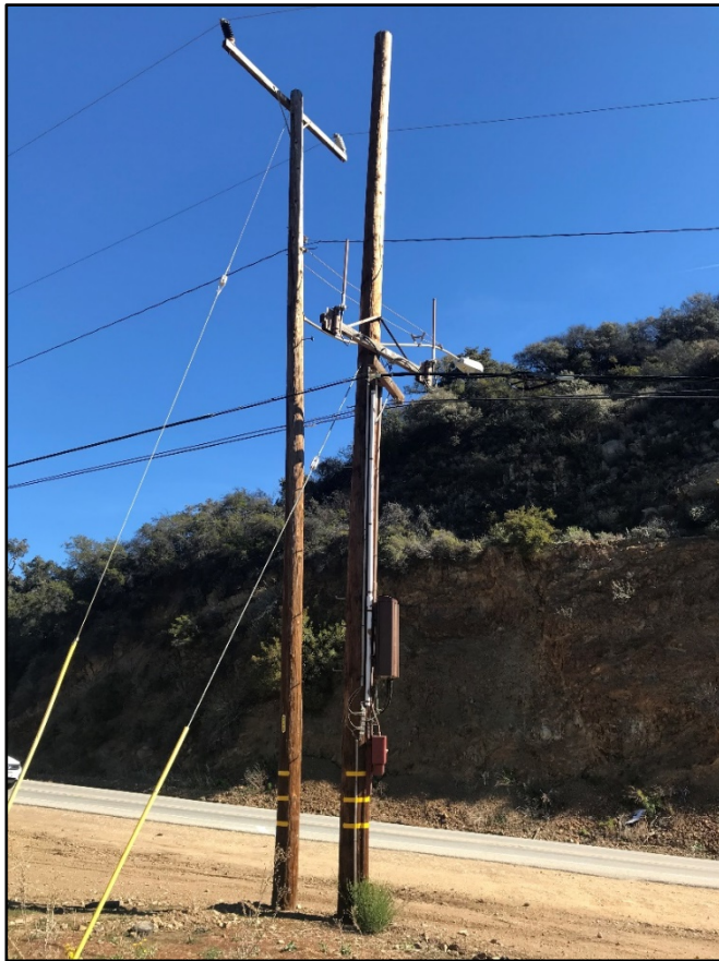
Figure 2. A commercial cellular antenna operating under a public road right of way at Santa Monica Mountains National Recreation Area. Source: OIG.
