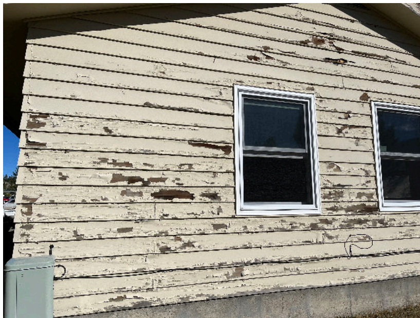
Example of failing lead-based paint, typical of “Lower Mammoth” housing in YNP. Lower Mammoth House 1, (photo from 2022).
