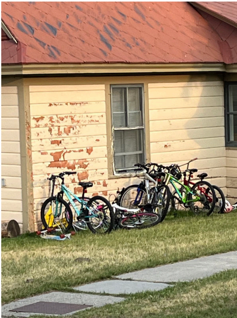
Yellowstone Home MA11, with peeling lead-based paint and children's bikes (photo from 2024).
