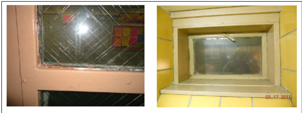
Figure 2-4b: Examples of Deteriorated Door and Window Glazing (NYCSCA, 2012)
