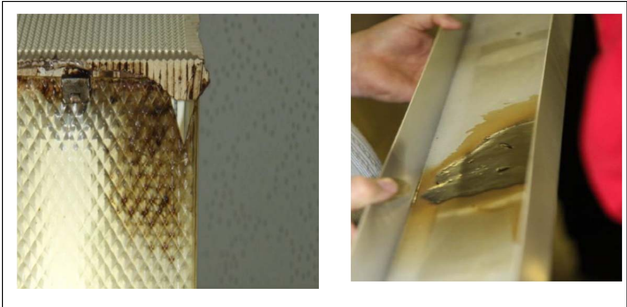
Figure 2-2e: Oily Stains on Lighting Fixture (USEPA, 2013b)
