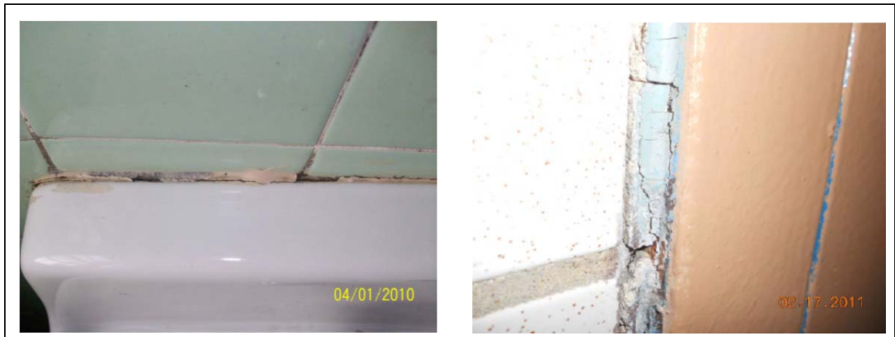
Figure 2-4a: Examples of Deteriorated Caulk (NYCSCA, 2012)
