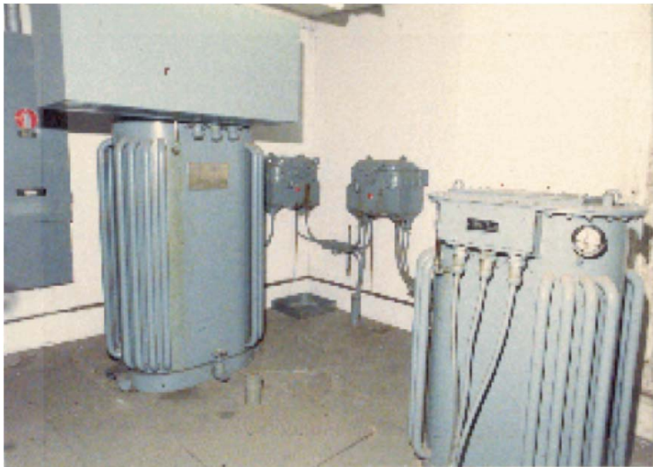
Figure 2-3: Example of Two PCB Transformers (USEPA, 2004)
