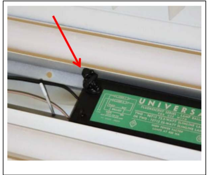
Figure 2-2b: Example of Material Leaking from FLB (USEPA, 2013b)
