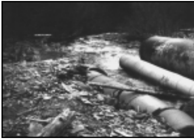
Major violation: water quality issues on Kennon Brook.
